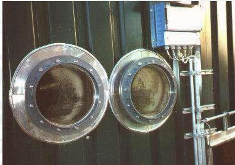
Control glasses for an industrial digester for solid organic waste, Germany [2]
